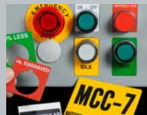
Control Panel Labeling
