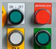
Raised Panel Labeling
