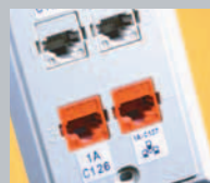
Patch Panel & Faceplates
