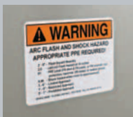
Arc Flash Labeling
