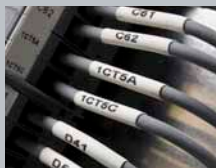
Wire & Cable Labeling
